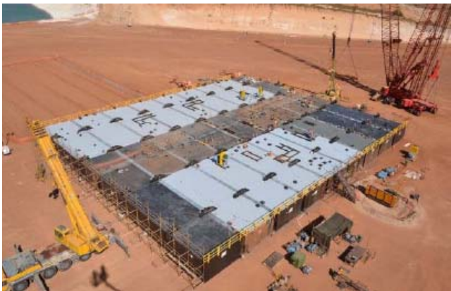
Spiral module pontoons (x18) of wet concentrator plant
