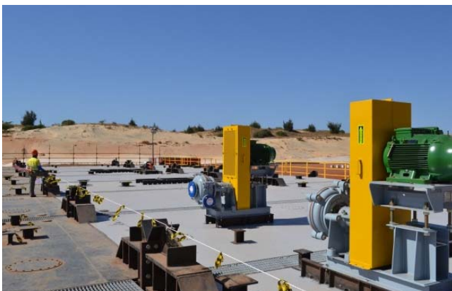
First pumps installed on the spiral module of WCP
